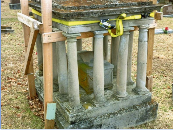
Paolini monument was crumbling and needed support braces to keep it from falling. (Nov. 2019)
