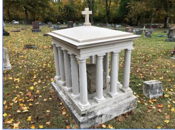
Paolini restoration required fabrication of 14 new limestone columns and a new roof. (Oct. 23, 2020)
